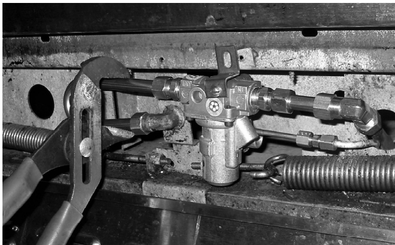
Installed Safety Valve. Tubing to orifice may be bent slightly with clamps to reach orifice.
