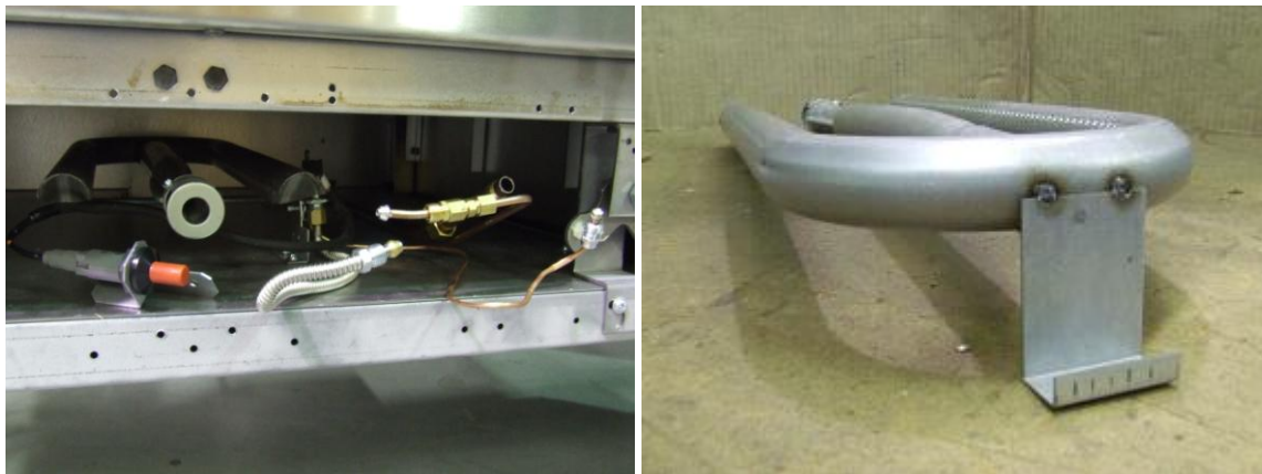
Left: Lower oven cavity after removal of front shields Right: Original burner with single welded bracket at end, will not be reinstalled
